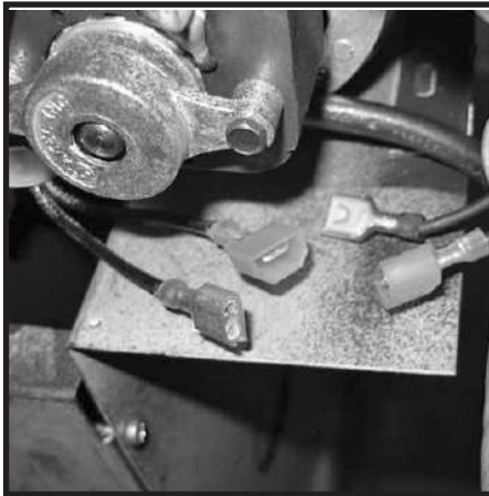
Figure 15: Disconnecting fan wires.
